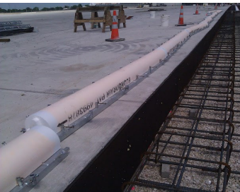
EPS forms with form release applied, laid out in numerical sequence and ready to be Installed.
