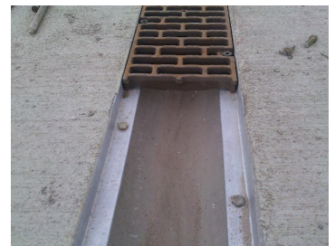
EPS forms are removed, the monolithic concrete trench is cleaned then install PT-2 grates with two point bolt down.
