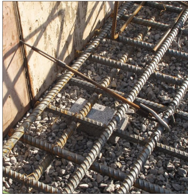
RH-48 Rebar Hooks and LCT-7 Turnbuckle ties used to tie Steel Ply edge forms to rebar mat on 20' x 30' x 3' slab pour.
